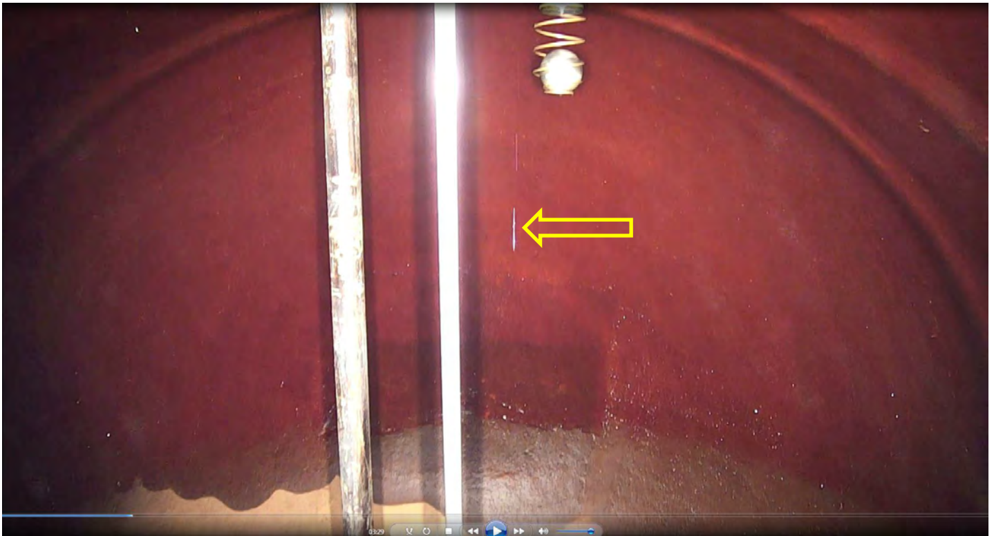
Figure 2-3: Drip falling from top of tank; possible moisture staining on end cap (03:29)
