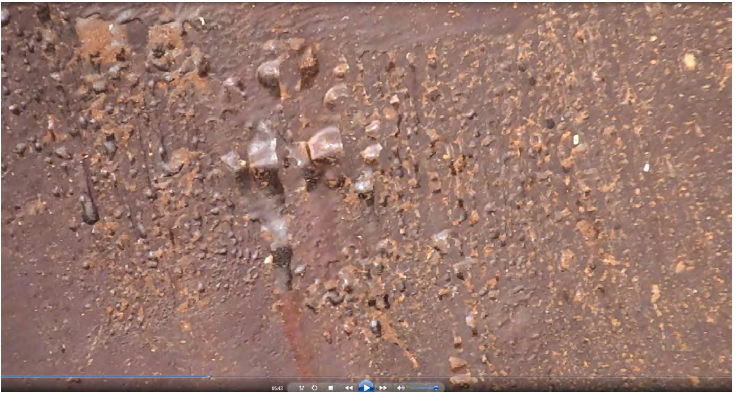
Figure 3-6: Possible peeling on tank wall (05:43)
