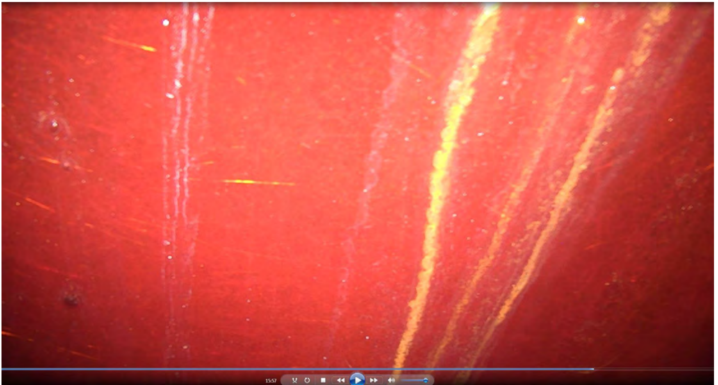
Figure 3-13: Staining on top of tank (15:57)
