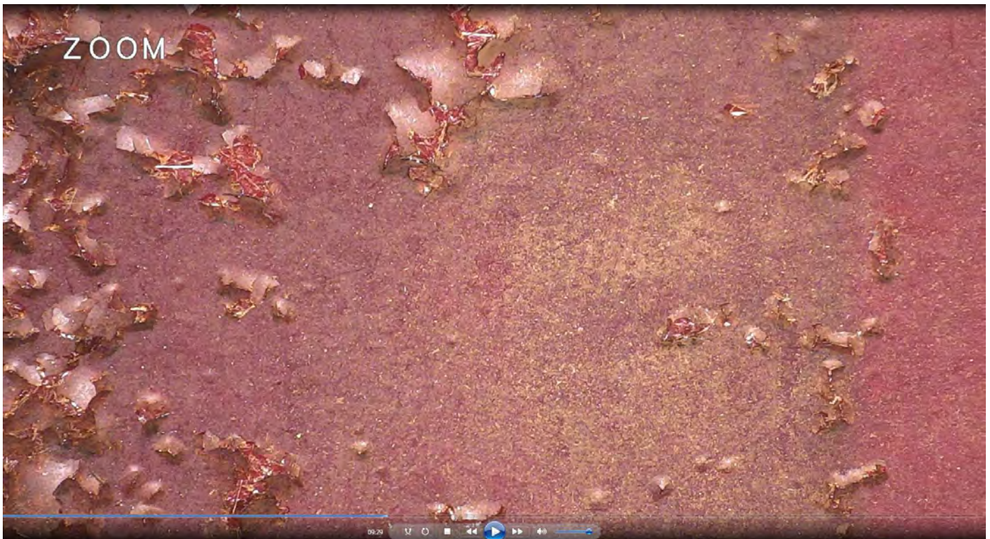
Figure 2-8: Flaking and peeling on tank wall (09:29)
