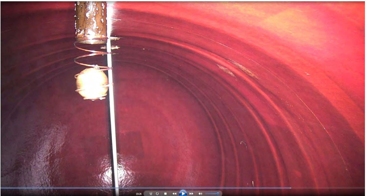
Figure 4-2: Corrosion on ball float assembly (19:26)
