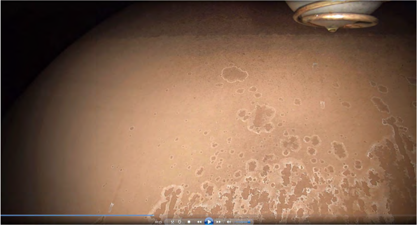
Figure 3-9: Staining on end dome; liquid drip on ball float (07:15)
