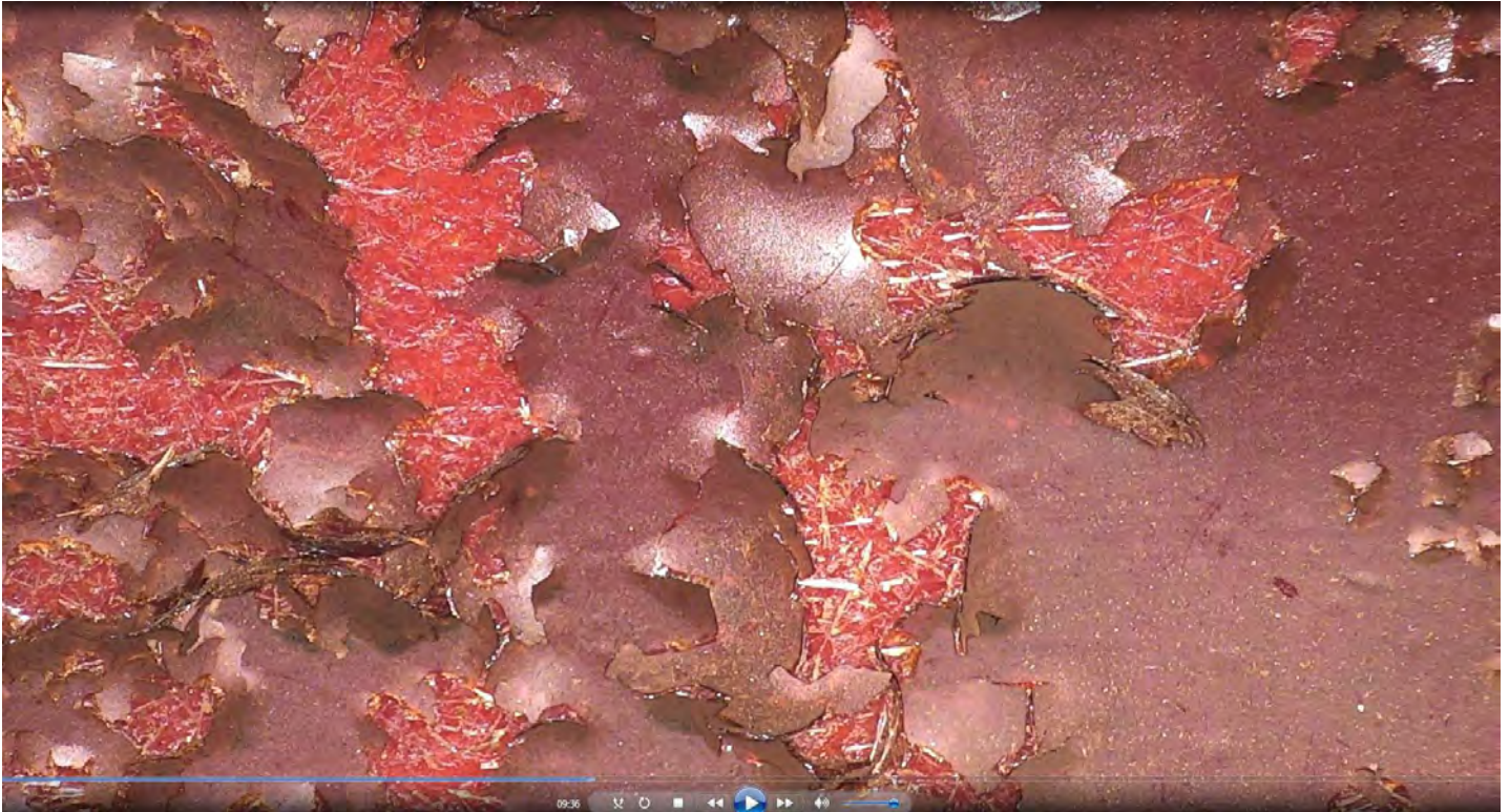
Figure 2-7: Close-up of peeling and flaking (09:36)
