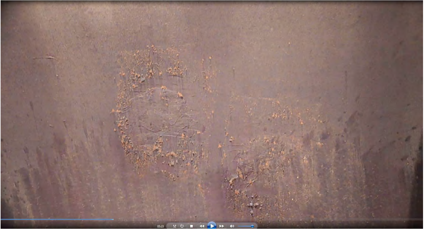
Figure 3-5: Possible peeling on tank wall (05:23)
