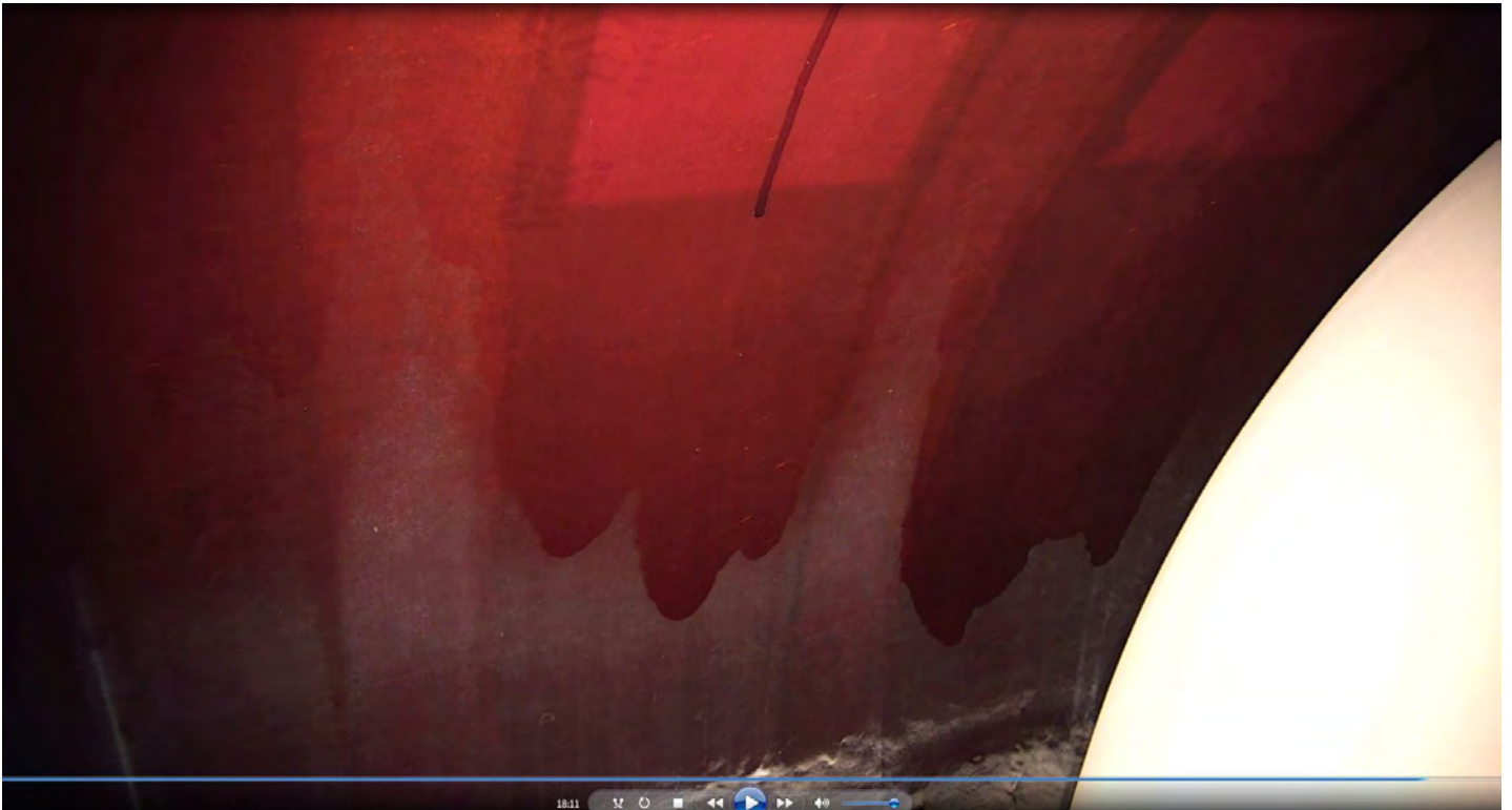
Figure 3-12: Discoloration on tank wall (18:11)
