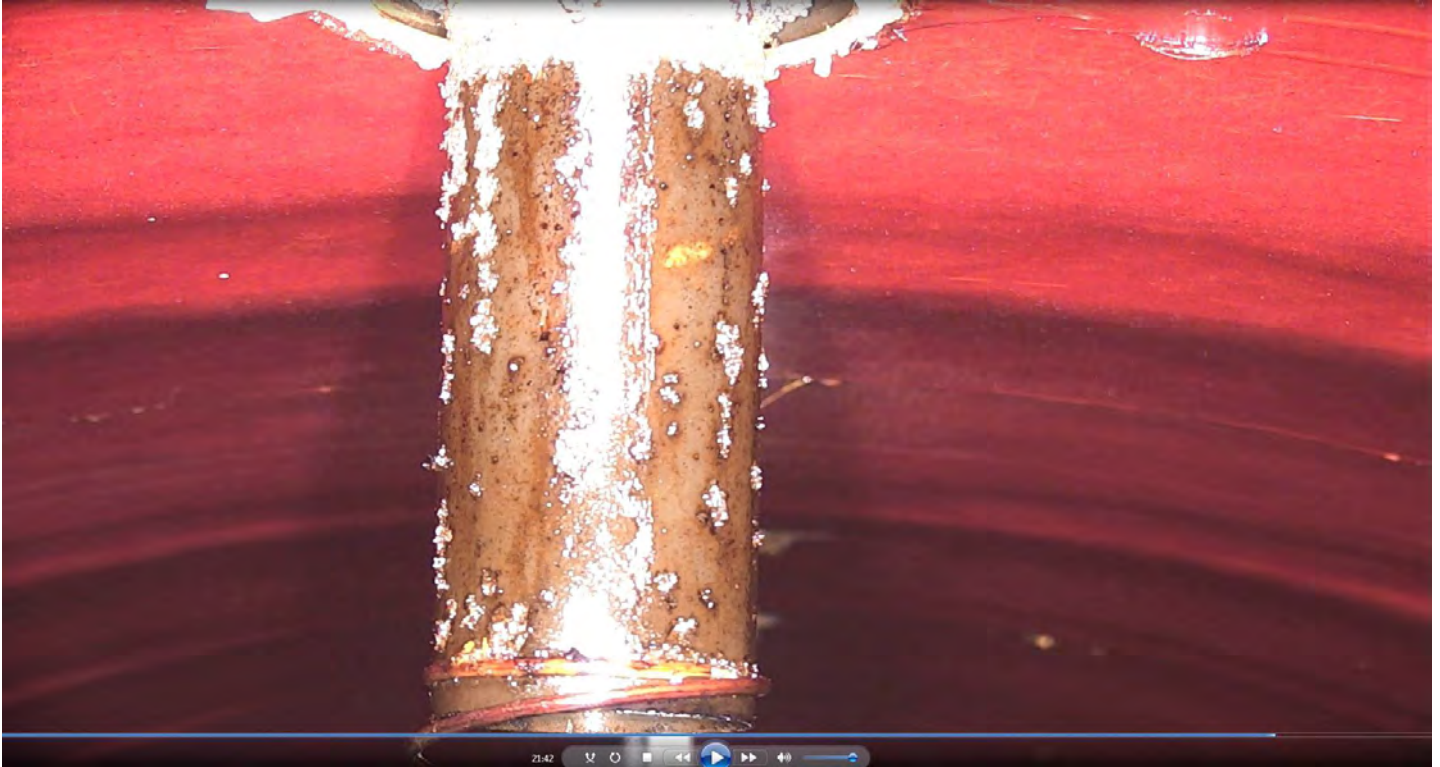
Figure 4-3: Corrosion on ball float assembly (21:42)
