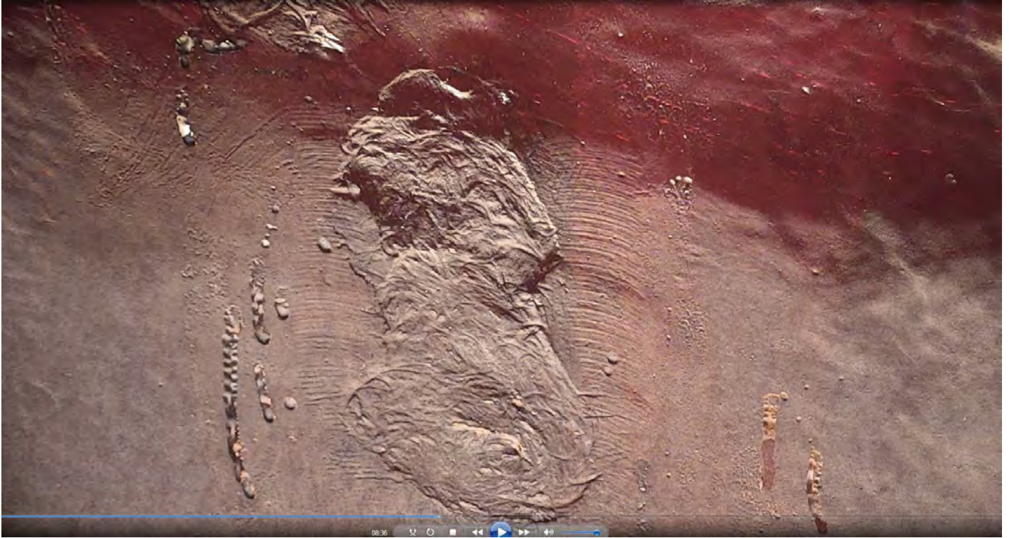
Figure 3-7: Possible patch on tank wall (08:36)
