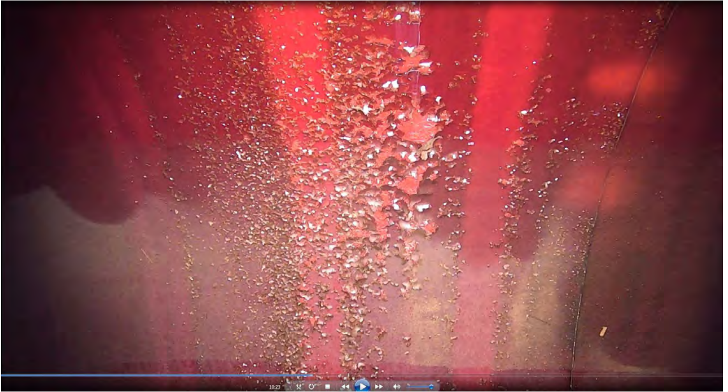
Figure 2-5: Flaking and peeling on tank wall (10:23)
