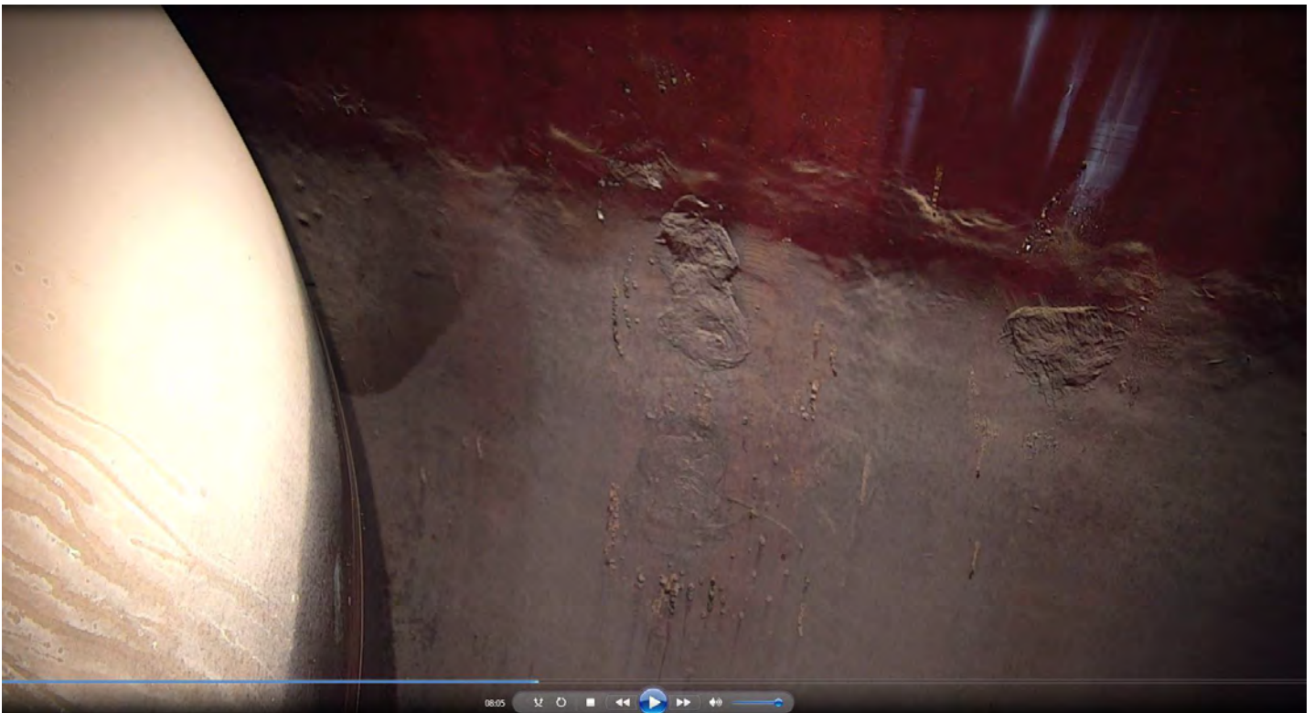
Figure 3-10: Possible moisture staining next to end dome (08:05)
