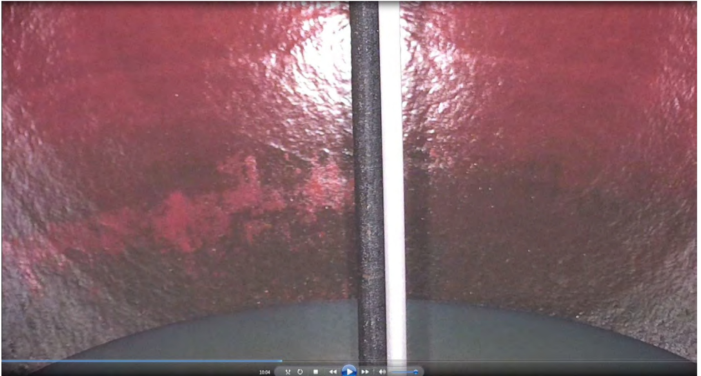
Figure 4-5: Possible corrosion on STP shaft (10:04)
