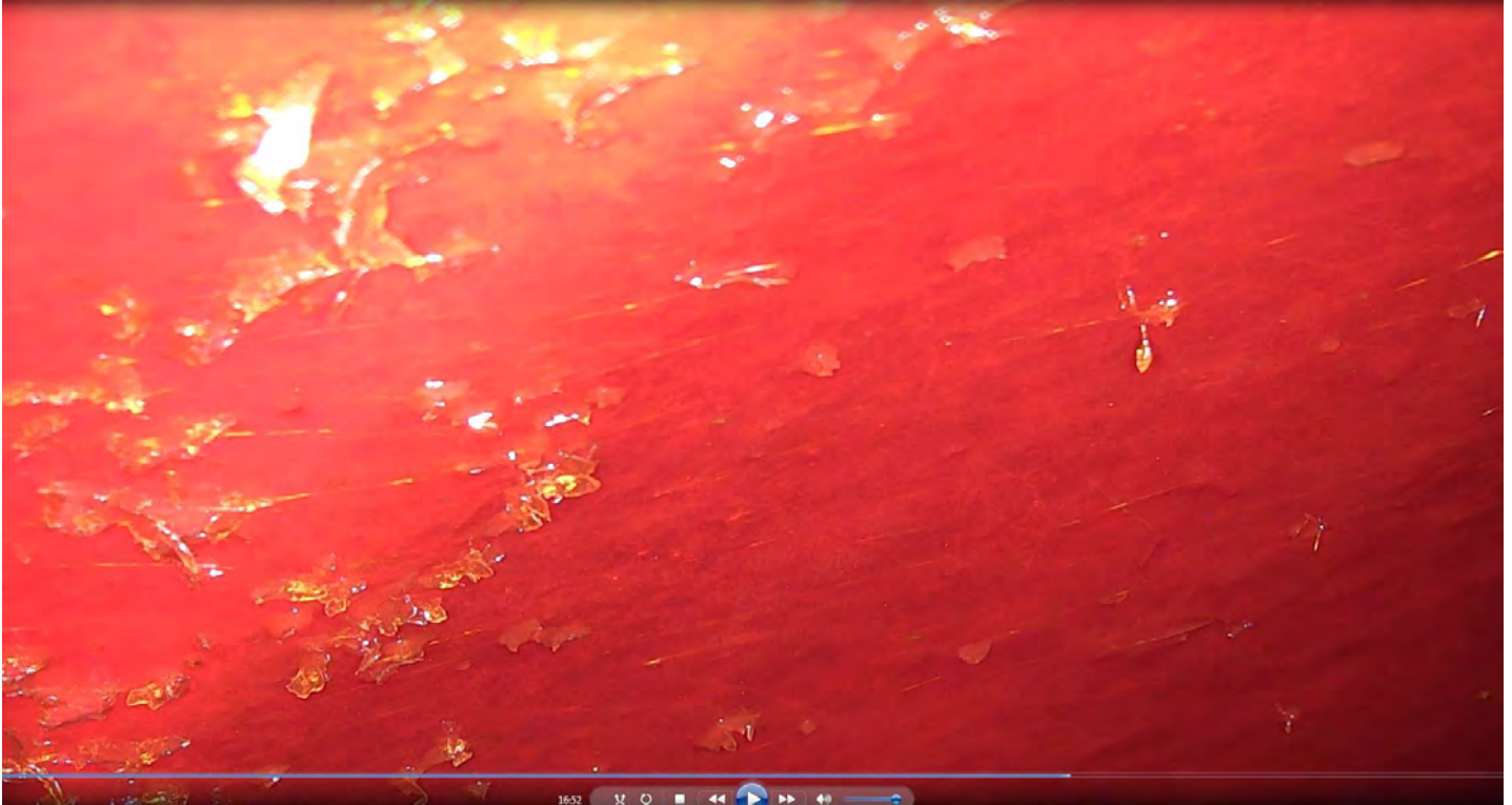
Figure 2-9: Flaking and peeling on top of tank (16:52)
